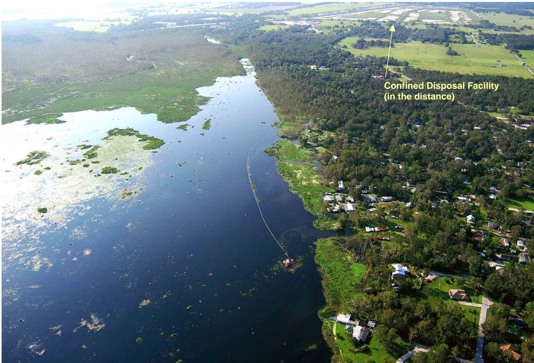
Aerial View of the Dredge In-lake Dredging Step 2 Near South End of Lake Panasoffkee
